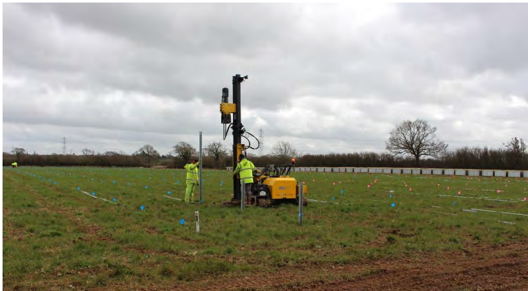
Plate 9a: Marking out location of the infrastructure and installation of PV module mounting structures (1 of 4)
