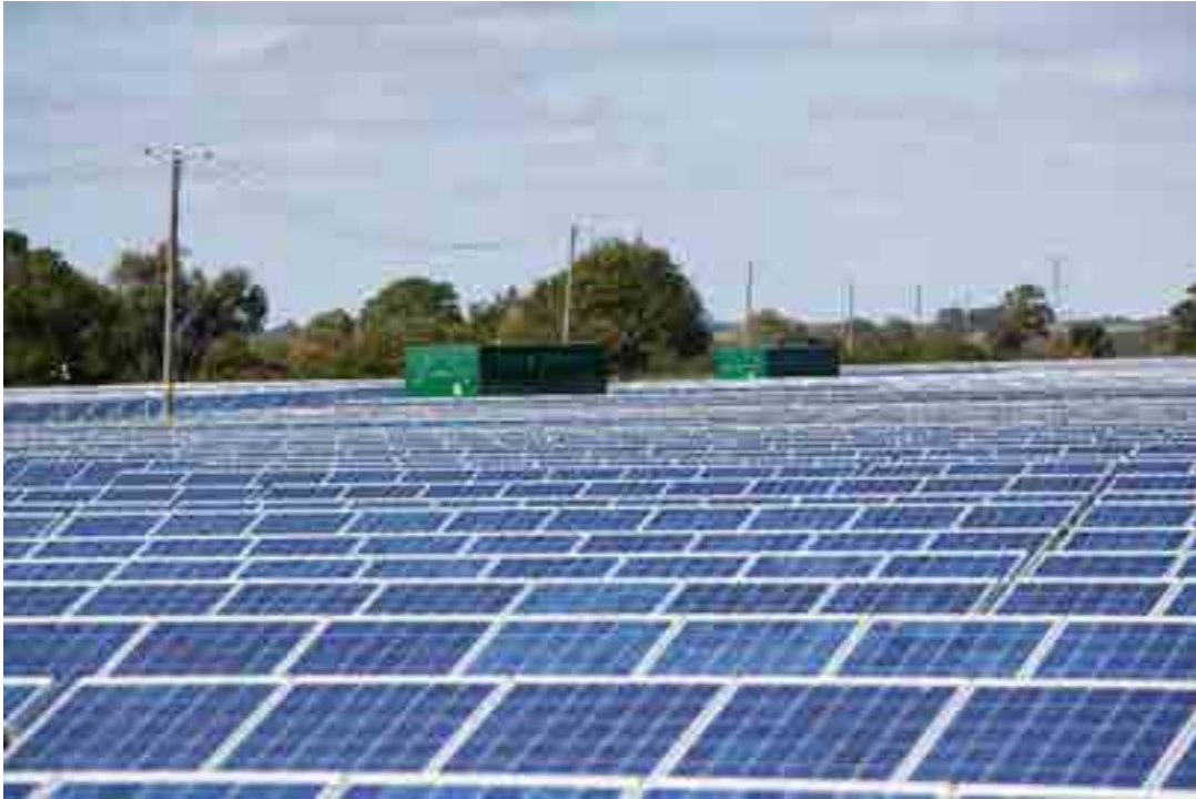
Plate 3: Example of Electrical Infrastructure Containers located within a solar array
